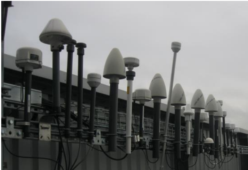
Fig. 29. View of GNSS antennas mounted on the roof of a critical infrastructure building. The inspection provides information on the number of systems dependent on GPS and the quality of the installation, as well as an insight into the period of origin of the individual GPS-dependent solutions. Source: own
