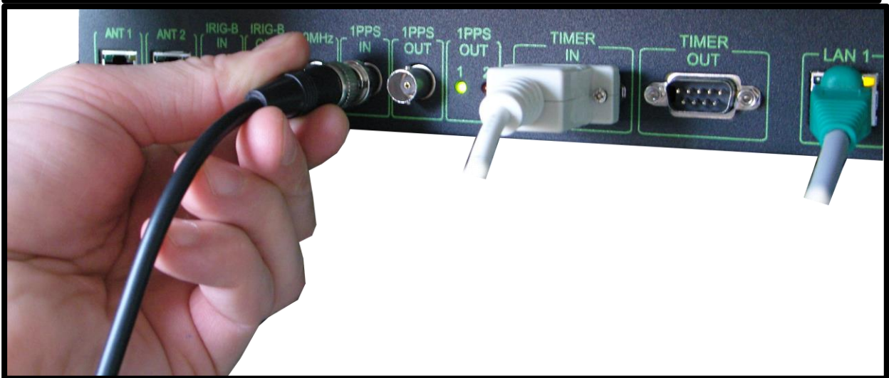
Connecting PPS (BNC) and ToD RS232 cables to NTS (the NTS-x000 back panel view)
